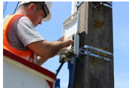
ACOME is a major player in overhead wiring and optical connection solutions.
